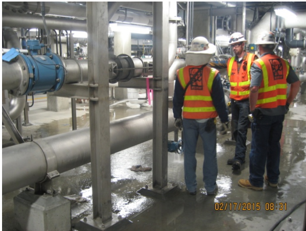
Feb 17 – Draining RO Unit F03
