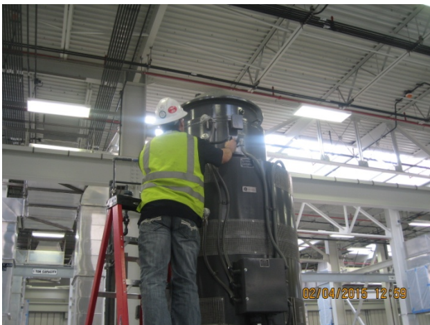
Feb 4 – Checking G02 RO Pump Vibration
