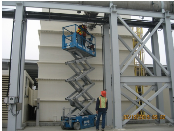
Feb 19 – Adjusting Decarb Inlet Valves
