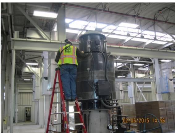
Feb 6 – Checking G03 RO Pump Vibration
