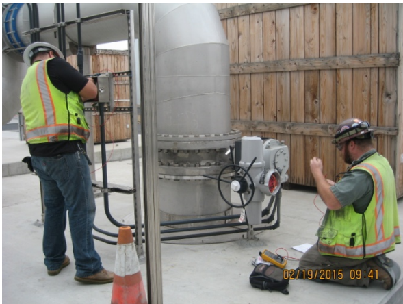
Feb 19 – Adjusting Decarb Bypass Valves
