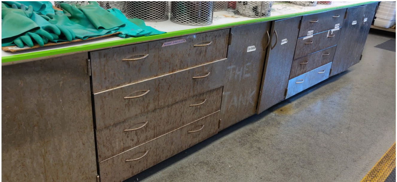
Photo 4: Rusting of cabinetry at center island utilized for storage and drying of cleaned glassware
