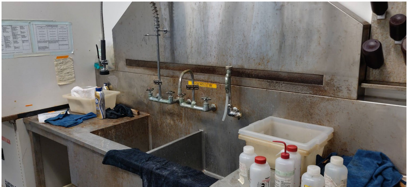
Photo 2: Rusting of fixtures and corrosion damage to faucets at second of three washing sinks
