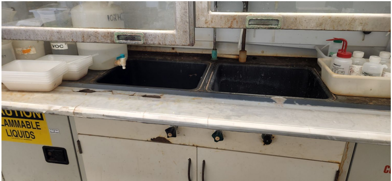
Photo 3: Rusting and corrosion of fume hood internal and external fixtures
