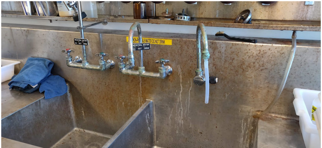
Photo 1: Rusting of fixtures and corrosion damage to faucets at one of three washing sinks
