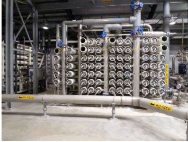
Existing RO System
