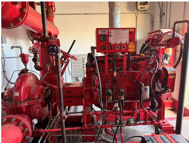
Figure 1 – Existing Fire Pump
