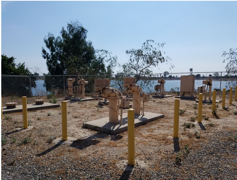
Figure 1: Existing Anaheim Lake Buried Valve Location
