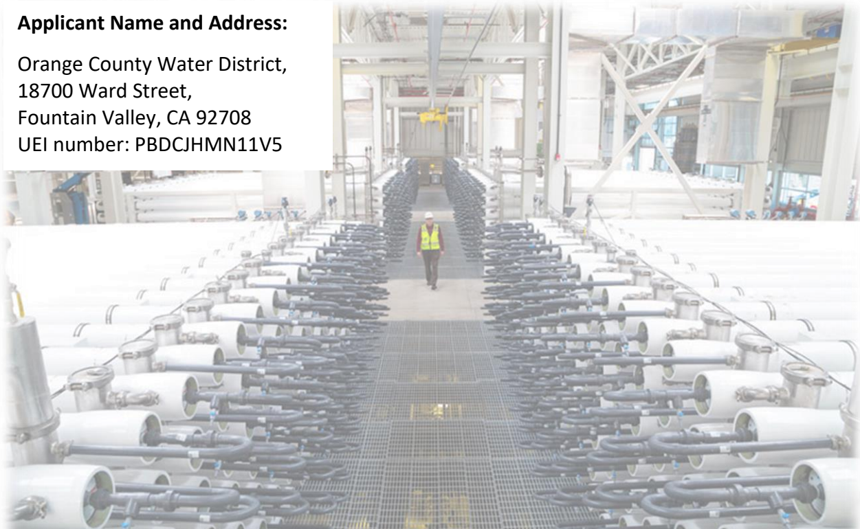
Picture: Advanced Water Purification Facility (AWPF), RO (Reverse Osmosis) Plant at Orange County Water District (OCWD)
