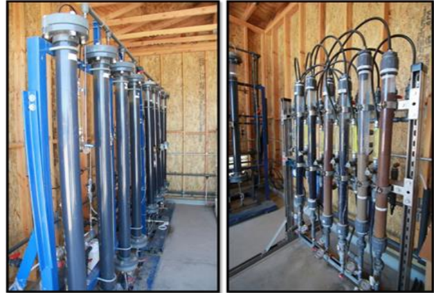
Figure 2. Drinking water wellhead PFAS treatment column pilot at OCWD
