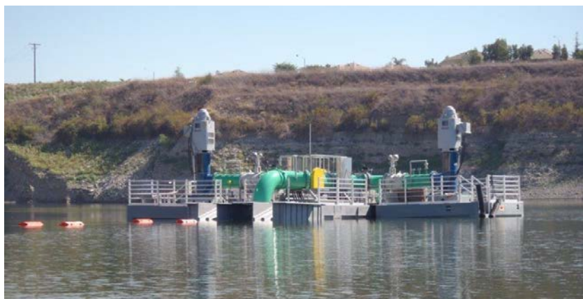
Figure 5-16: Santiago Basins Pump Station
