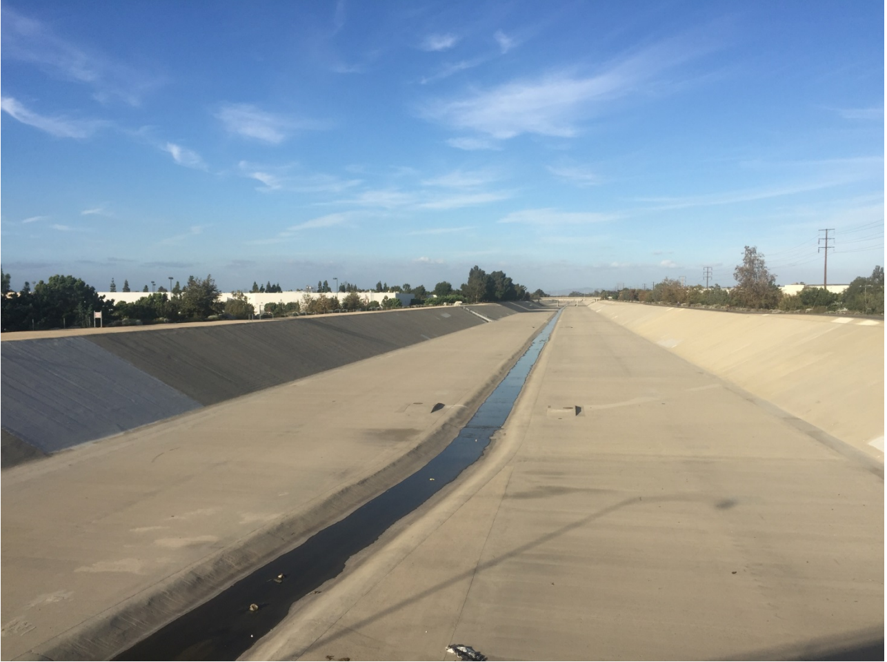
Figure 3-28: Santa Ana River View upstream from Talbert Avenue Bridge in Fountain Valley. The portion of the river here has both concrete levees and bottom.
