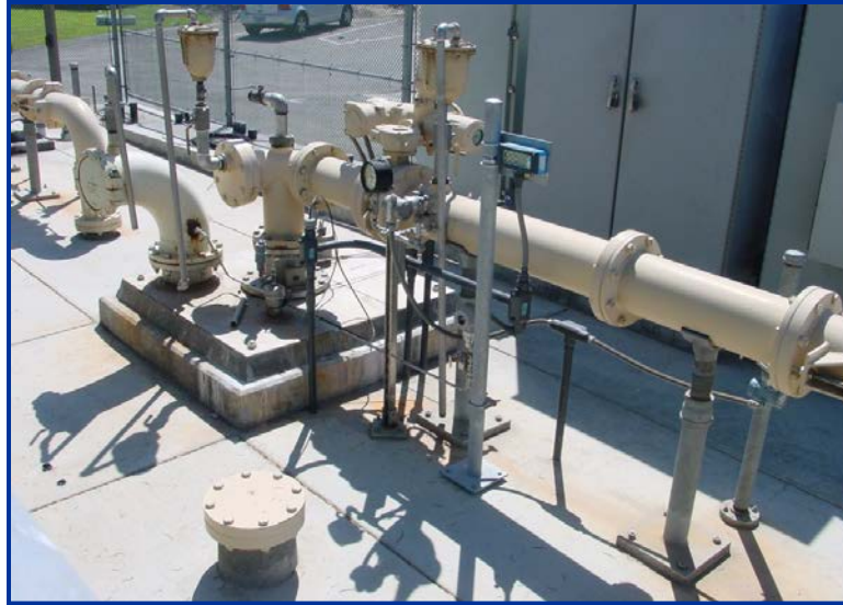
Figure 3-3. Modern Injection Well Site OCWD-I26
