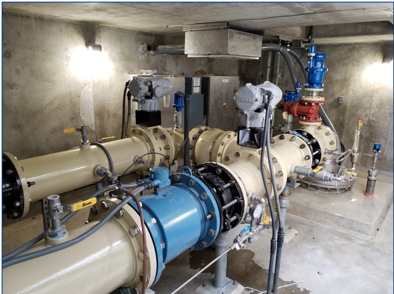
Figure 7-3. MBI Centennial Park Injection Well
