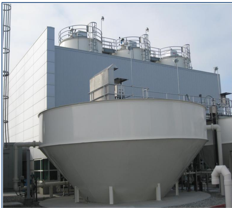
Figure 2-16. Lime Post-Treatment System
