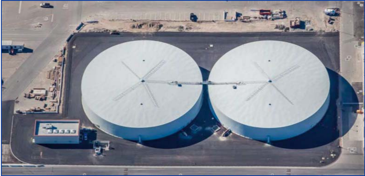
Figure 2-3. OC San Plant 1 Secondary Effluent Flow Equalization (SEFE) Tanks and Pump Station
