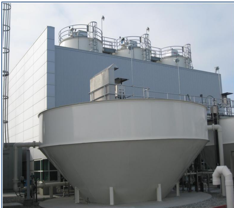
Figure 2-24. Lime Post-Treatment System
