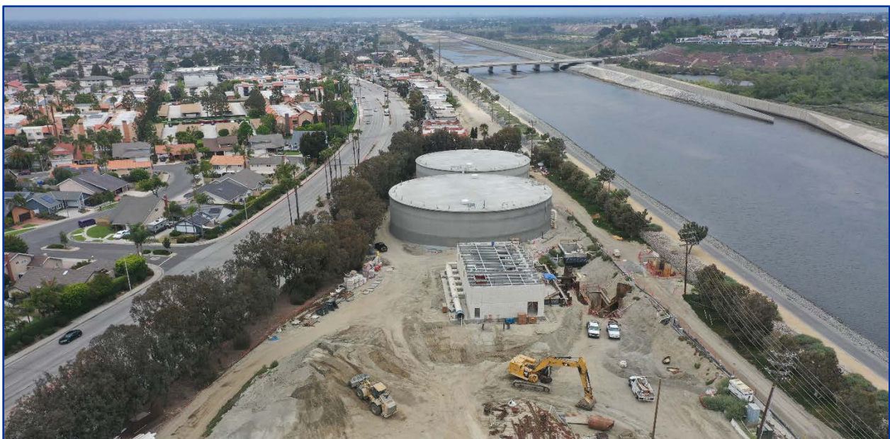
Figure 2-4. OC San Plant 2 Secondary Effluent Flow Equalization (SEFE) Tanks and Pump Station
