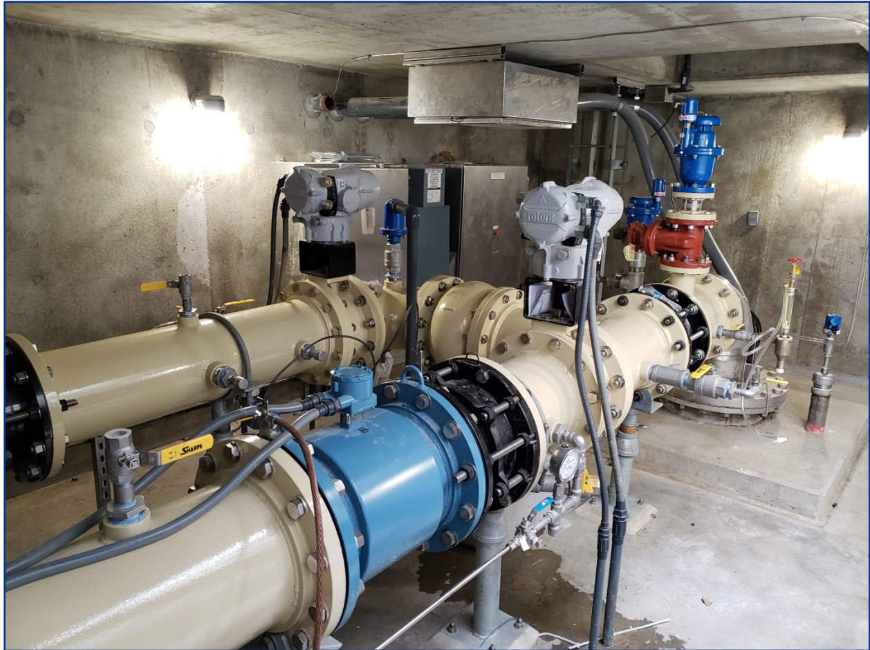
Figure 7-3. MBI Centennial Park Injection Well
