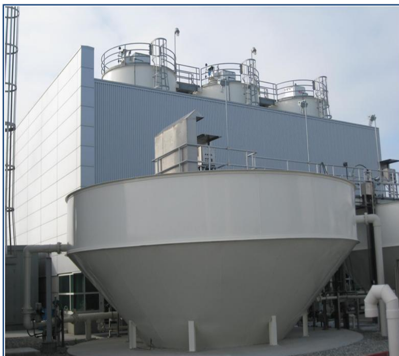
Figure 2-16. Lime Post-Treatment System
